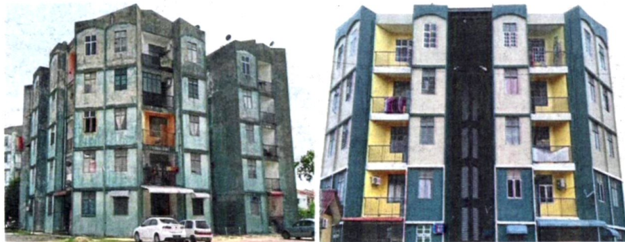
The repainting work of Bandar Baru Kubang Kerian Apartment in Kota Baru is among the many maintenance projects under the TTPM - before (pic left) and after (right).
